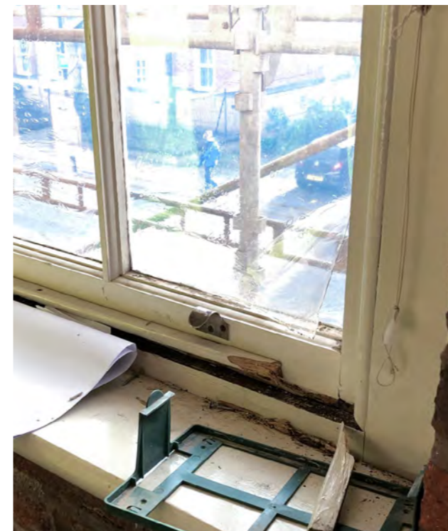
Above: damaged sash window
