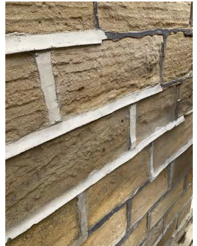
Above: Poor quality pointing
